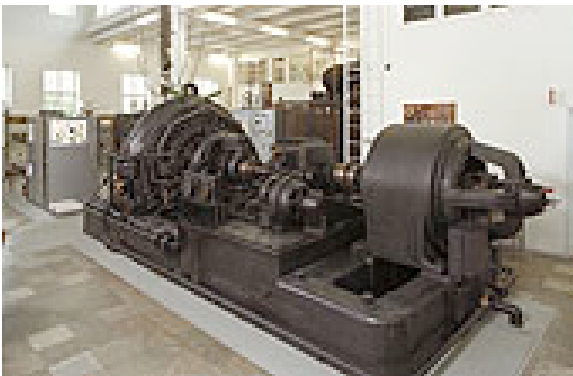
The Alexanderson generator
